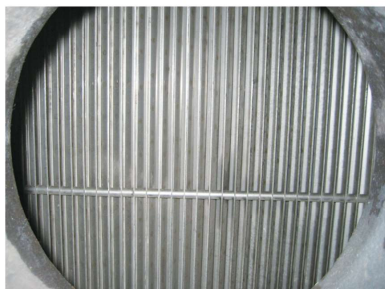
安装在设备内的环形叶片 Circular Vane Installed in the Vessel
