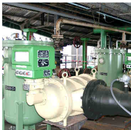
Ship loading skid
