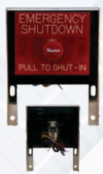
Electric ESD Station
